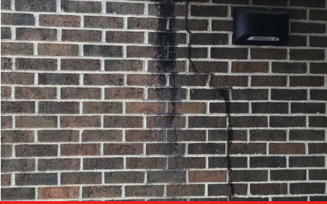
Aged masonry on both buildings needs repair due to water infiltration.
