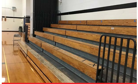
The 1996 high school bleachers are inadequate and unsafe.
